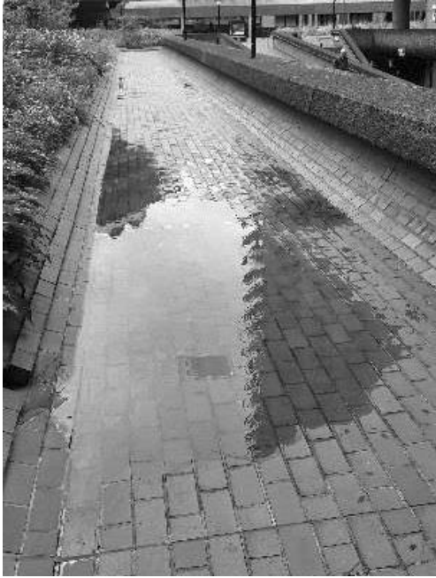
Flooding on the new Beech Gardens Highwalk
