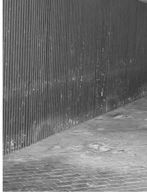
Railings unpainted for at least 20 years and 20 mm thick calcination on Defoe Place
