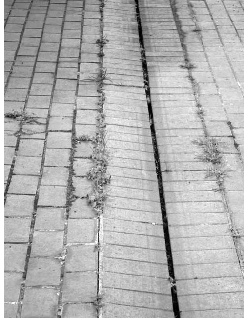
Plants in mortar joints on Cromwell Highwalk
