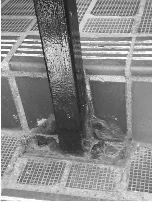
Corroded fixings on steps up to Beech Highwalk from Lauderdale Place
